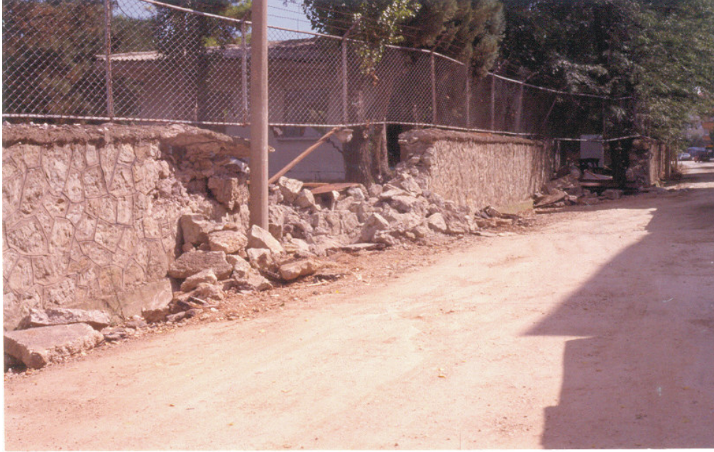
Figure 13. Stone wall of the Navy base at Stop 2 displaced 4.30 m in a 50 m width of deformation zone in the 1999 İzmit earthquake.
